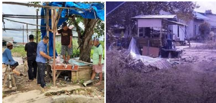
Figure 7. The men installed the stilt space as a communal space etc (left), and the stilt room was completed (right) (Source: author).
