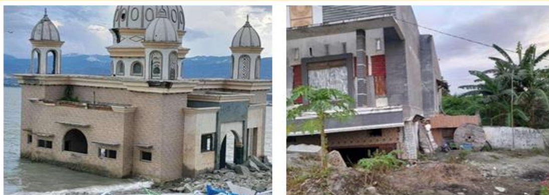
Figure 1. (a). The tsunami damaged the mosque; (b) Houses sank into the ground due to liquefaction. Documentation by Team
